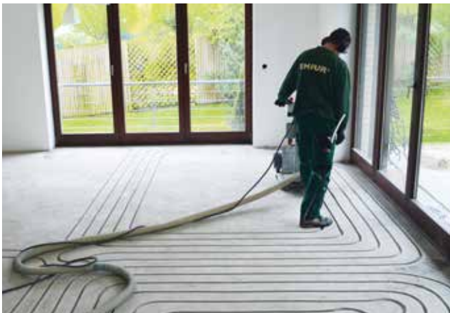
Virtually dust-free cutting of the grooves into the existing screed by an experienced installation team according to plans.
